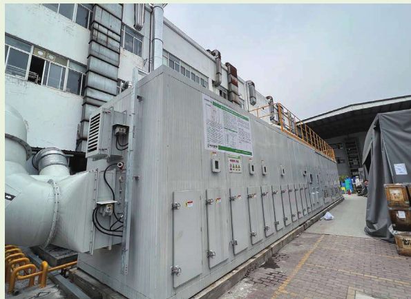
Installation of the RTO waste gas treatment equipment in progress RTO蓄熱式氧化廢氣處理設備安裝建設中
